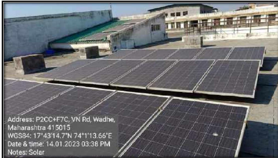
Fig. 7.1.3.9. Solar Energy Panel
